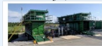
Direct Air CO 2 /Capture Skid
