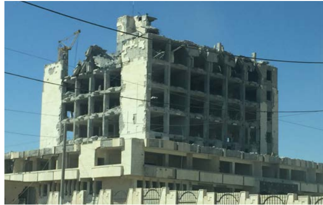
Figure 1. Original Tabqa Hospital, which was turned into an ISIS C2 center. Tabqa, Syria, 2017.
