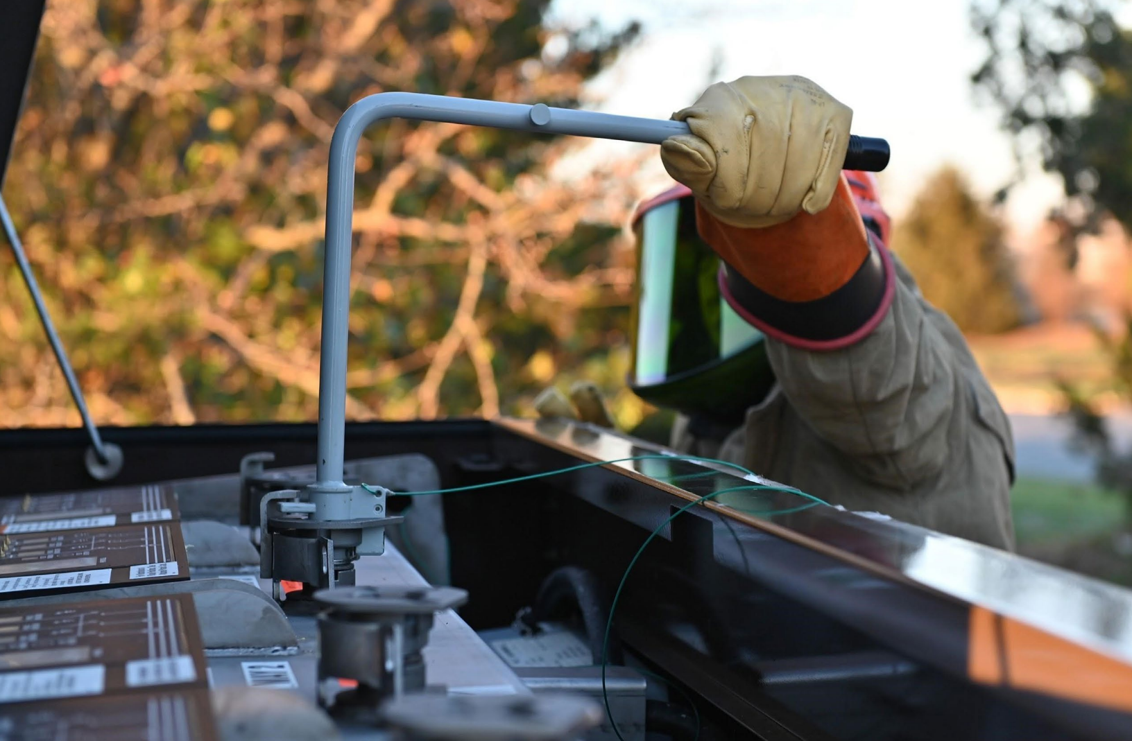
Personnel prepare to shut down electrical power to a military base during an ERRTX in November 2020.
