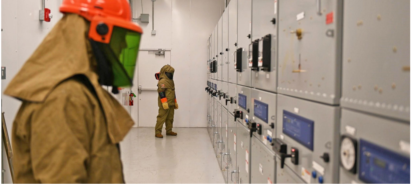
Civil Engineering Squadron personnel prepare to shut down electrical power during an ERTTX, 19 November 2020.
