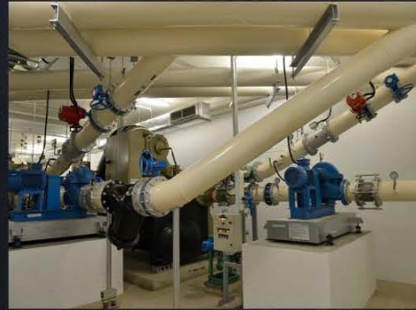
Big pipes, small pumps
