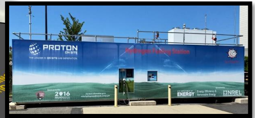
120 kW PEM electrolysis/refueling (40 kg/day)
